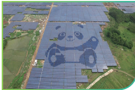
Located at Guigang, Guangxi, our second Panda Power Plant has a total installed capacity of 60MW. 第二個熊貓電站落地廣西貴港，總裝機容量為60兆瓦。
